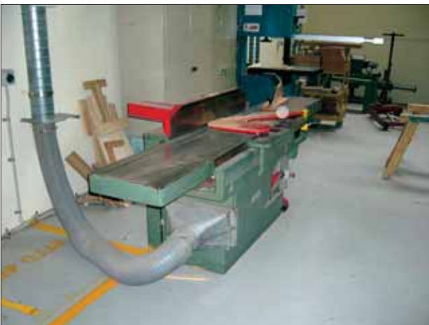
Woodworking dust generated by a buzzer is extracted via forced extraction and ventilation.
