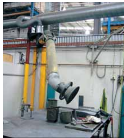
Welding fumes are extracted via flexible locatable, extraction system.
