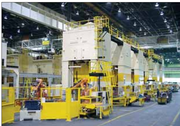
Permanent gantries, ladders and walkways are incorporated into this machinery and equipment to reduce the risk of a fall from height during operation and maintenance.
